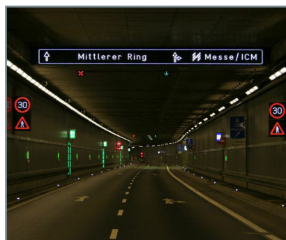
Variable message sign, speed limit and warning signs
